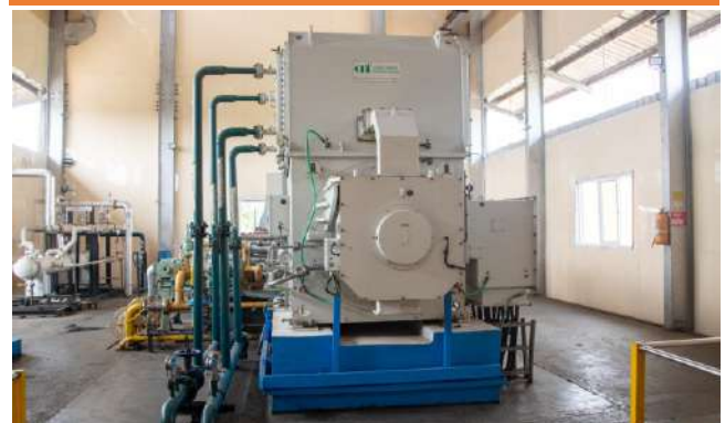
OUR 5 MEGAVOLT - AMPERE (MVA) TURBINE AT THE MAIN ESTATE INSTALLED IN 2021
