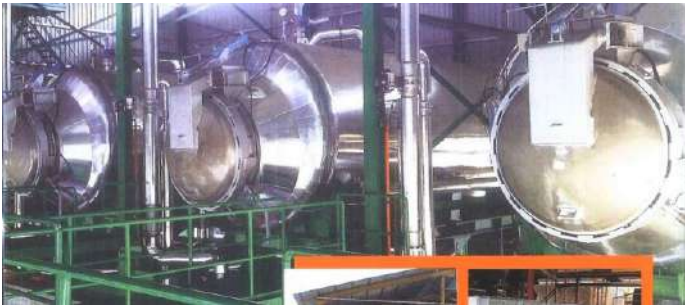
FIRST EVER TILTING STERILIZER IN AFRICA INSTALLED IN OUR MAIN ESTATE OIL MILL
